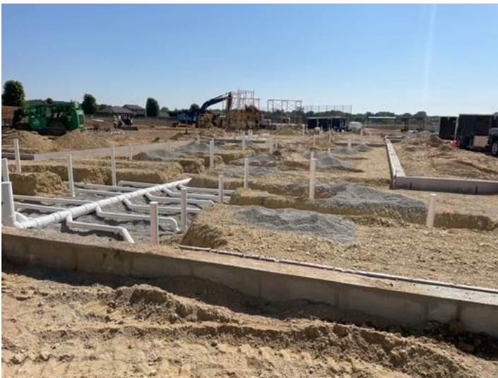
Underground plumbing Bath House interior Taken on Jun 9, 2023, 10:04 AM CDT Added on Jun 9, 2023, 11:01 AM CDT Added by andrew gordon
