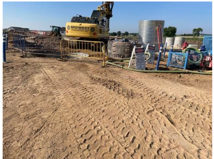
Drilling for the Underdrain Taken on Jun 9, 2023, 8:26 AM CDT Added on Jun 9, 2023, 9:01 AM CDT Added by andrew gordon
