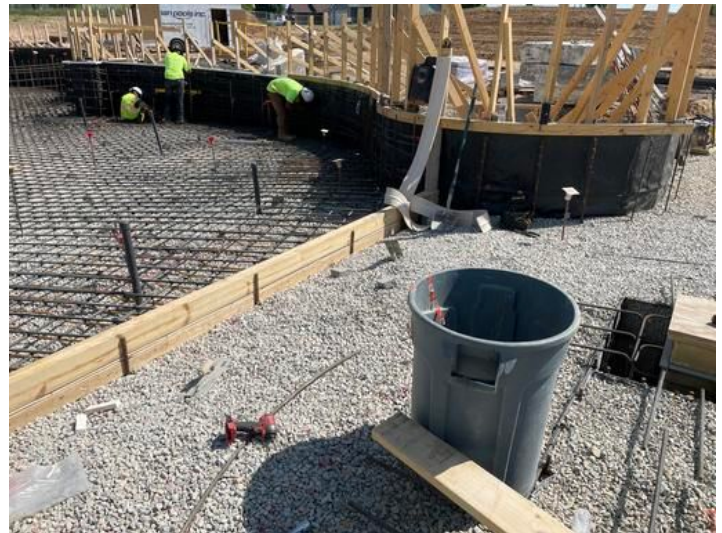
Rebar installation at "Lazy River" pool Taken on Jun 9, 2023, 10:05 AM CDT Added on Jun 9, 2023, 11:01 AM CDT Added by andrew gordon
