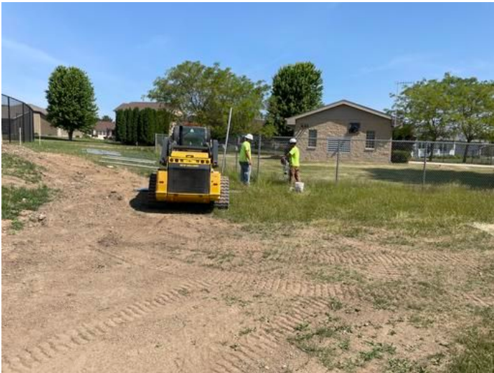
reinstall fencing around existing pump house Taken on Jun 9, 2023, 10:29 AM CDT Added on Jun 9, 2023, 11:02 AM CDT Added by andrew gordon
