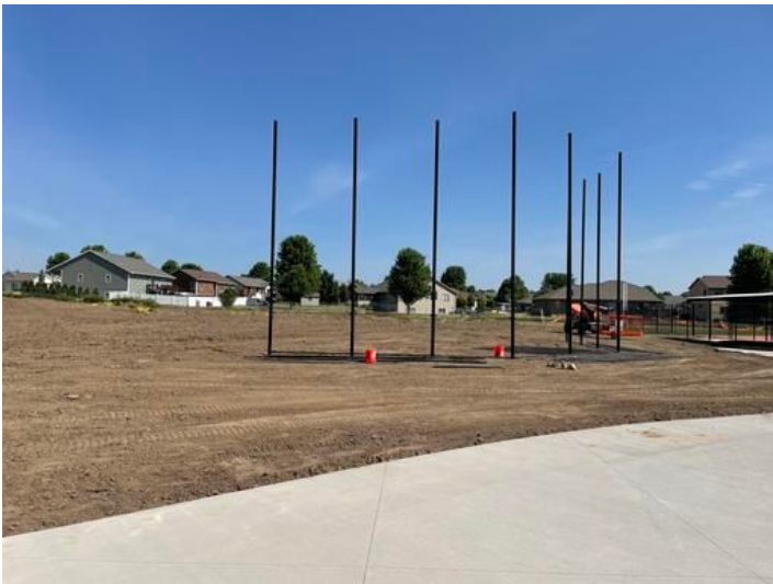
Start on Backstop fencing Taken on Jun 9, 2023, 10:09 AM CDT Added on Jun 9, 2023, 11:01 AM CDT Added by andrew gordon
