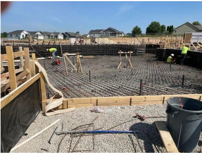
Rebar at "Lazy River" pool floor Taken on Jun 9, 2023, 10:05 AM CDT Added on Jun 9, 2023, 11:01 AM CDT Added by andrew gordon
